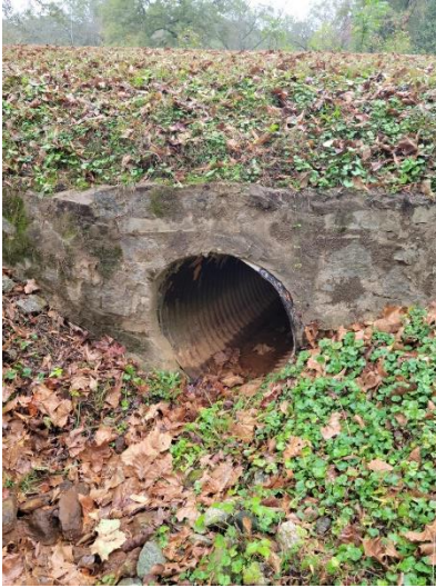
Turkey Creek on W. Soule Street - 36" Steel Pipe that is approximately 40 years old.
